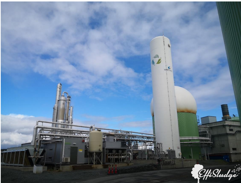
Figure 4 – Gas upgrading and LBG storage.
