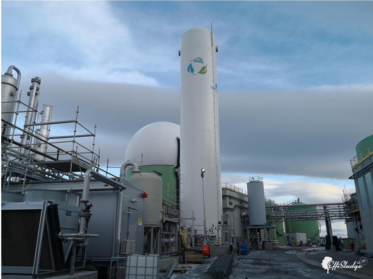
Fig 3 – From the left: upgrading units, secondary digester with gas holder, LBG storage tank (white tank with BK logo), machinery house with centrifuges, piping to/from digesters.
