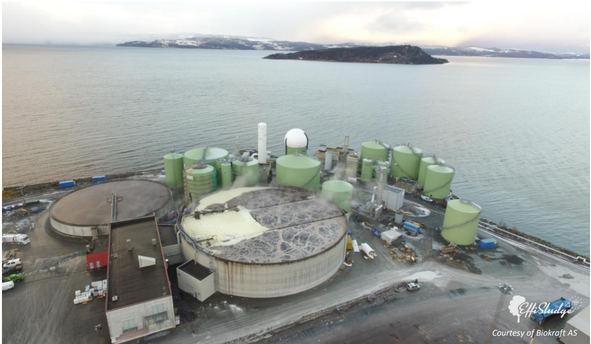
Fig 1 – Aerial overview (January 2018) of the construction site with existing wastewater treatment plant (circular basins).
