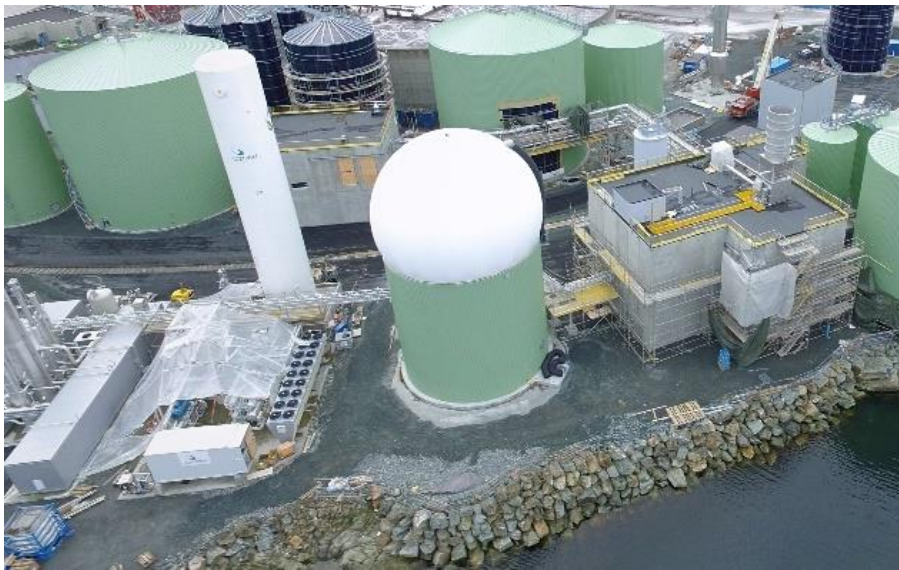
Figure 4 – Overview of secondary digester (with white gas holder) and gas upgrading unit (with LBG storage tank).
