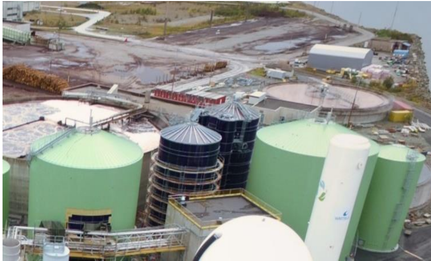
Figure 5 – Overview of two main CSTR digester (completed) and under construction ECSB units (black tanks).
