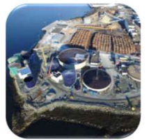
Pilot (top) and WWTP with AD plant under construction site at Skogn (bottom).
